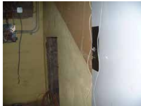
Wall on the steps to the basement had been expanded to the meet the first floor of the building.
