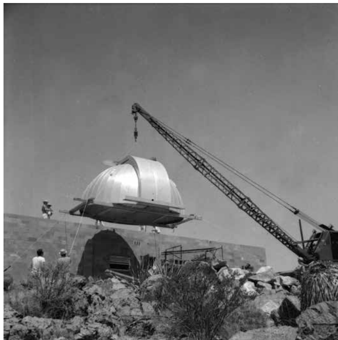
Lifting one of the domes onto the top of the building in 1964. Photo courtesy of University Archives.
