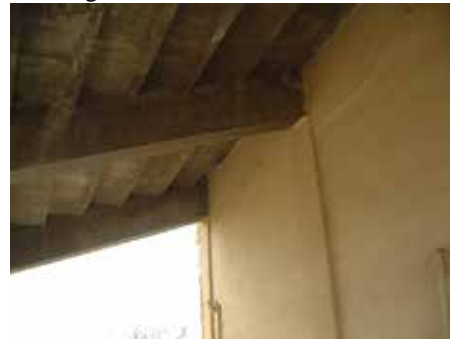
Underside of the bleachers that were thought to be connected to the main part of the building.
