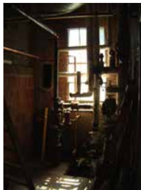
Mechanical Room showing old plumbing fixtures.
