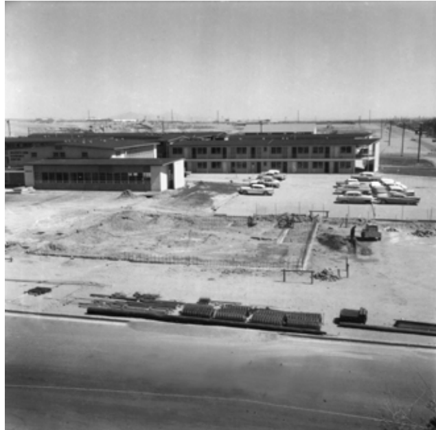
Laying the foundation for the new post office in 1965. Photo courtesy of University Archives.
