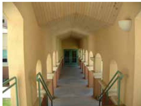
Inside the walkway that connects the southwest wing to the original building.
