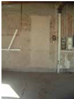
Southern entrance to the original laundry facilities that has been bricked up.
