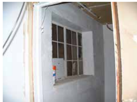
Basement window that had once been visible from the exterior of the building. There is approximately a foot of space between it and a cinderblock wall that encases the window.
