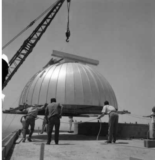
Setting one of the domes into place on the roof in 1964. Photo courtesy of University Archives.
