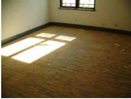
In a room in the north wing of the building, the hardwood flooring is covered in adhesive that used to secure flooring that had been laid over it.
