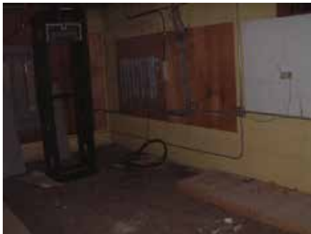
Telecom room located in the basement.
