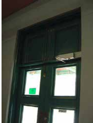
The original front doors were cut off at the top panels.
