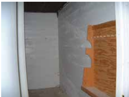
Old rack for shot guns that was left behind in a basement room by the police department when they moved out.
