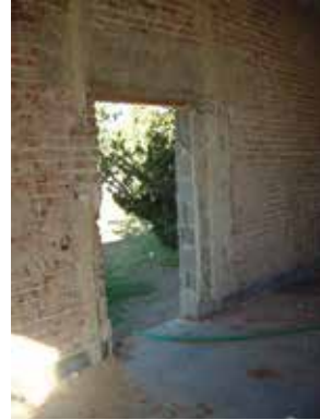
The original west Entrance. Cinder Block is visible where the door way was narrowed from two doors to one.
