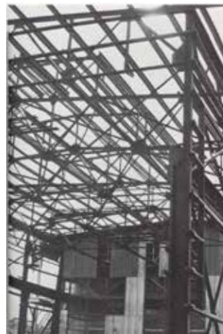
Photo from the 1971 yearbook. The Caption reads, "So too, Foster Hall was added on to. Foster Hall, one of the oldest buildings on campus still in use today, is the home of the Biology Department. But what will this addition do to the Bio. 110 lectures?"
