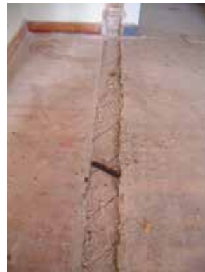
Underneath the carpet that covered the floor while the police department occupied the building, is hardwood flooring and sub flooring that is still in fairly good condition.
