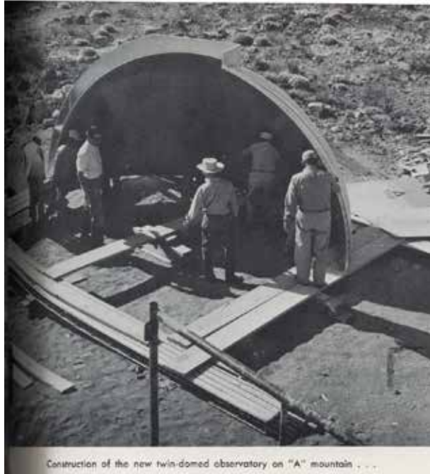
Photo from the 1964 yearbook. Caption reads, "Construction of the new twin-domed observatory on "A" mountain ...".
