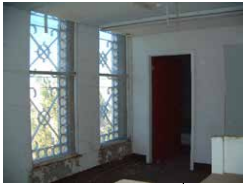
Room on the west side of the 3 rd floor that leads to the spiral stairs to the 5 th and 6 th floors of the tower.
