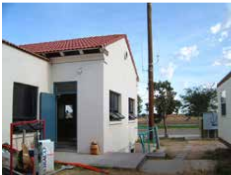
Picture features northern access door and the outside steps to the basement.
