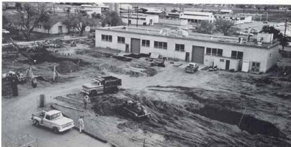
Construction on the eastern wing of Jett Hall, and Jett Annex. Photo from the 1966 yearbook.
