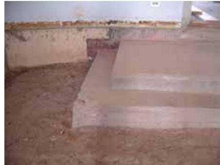
Edge of steps that had originally been located in the original western exterior (eastern end of west wing addition) of the building.
