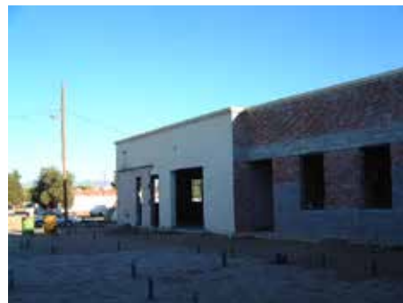
Soil has been built up to the level of the thresholds of the north entrances to the building to support the new addition.
