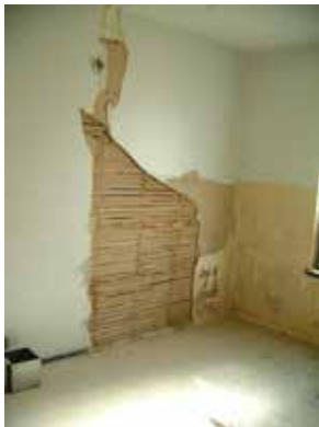
Plaster walls in the bathroom located at the end of the north wing.
