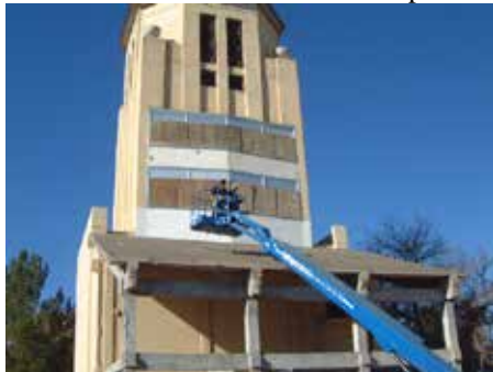
The only access to the top part of the tower was by taking a boom lift to the top of the bleachers.
