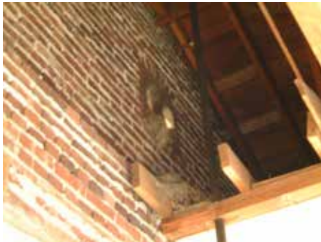
Bird nest on the interior side of the brick exterior west wall's gable roof end.
