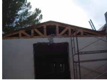
End of the west wing that has had a doorway punched through the exterior wall of the addition to allow passage to an additional addition to the west wing.
