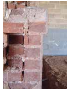
Section of the exterior wall of the dining hall. Shows the original brick with a coating of stucco.
