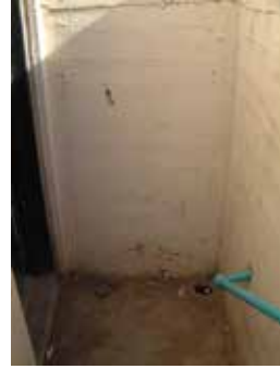
At the bottom of the exterior steps to the basement, there is evidence of an opening that had been filled in with cinderblock.
