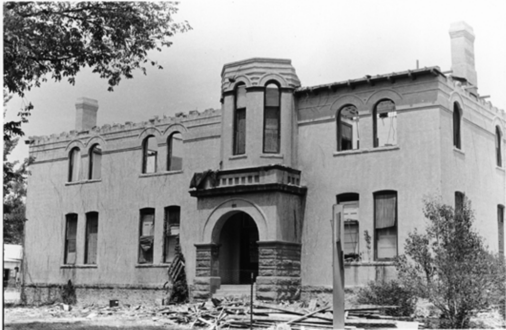
Photo of the building being torn down in 1974. Photo courtesy of University Archives.
