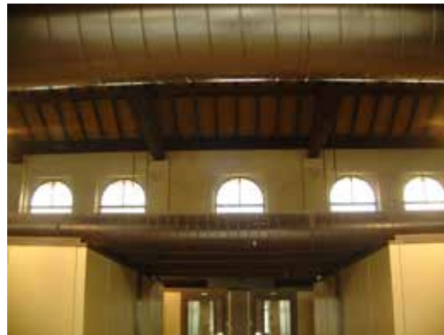
HVAC systems span across the tops of the practice rooms.
