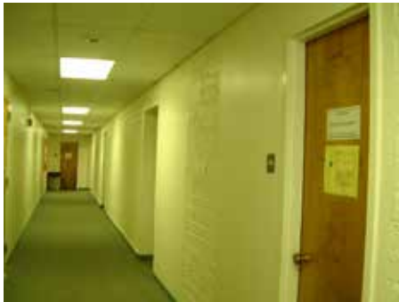
South hallway that shows rough brickwork that may have been an exterior wall at one time.
