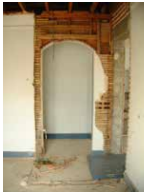
Arched doorway that used to lead to the basement stairs. The wall surrounding it features what is left of the plaster and slat walls that were original to the building.
