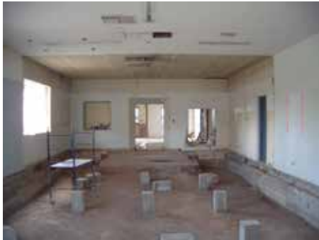
East wing of the building. The rectangular blocks of concrete are footings that supported the floor. The floor had also been laid over the original steps on the exterior of the building.
