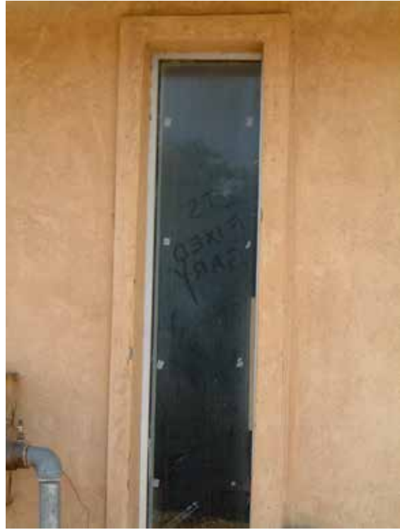
Window on south side of building with the message "Its Fixed Gary." The message has been there for several years.
