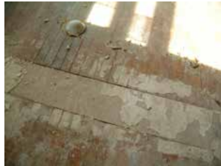
Section of flooring in the main lobby where a section had been patched where a stud wall had been removed.
