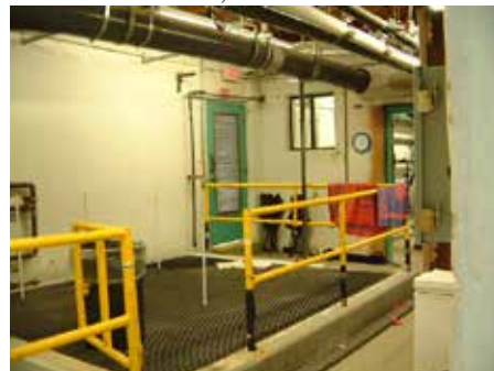
Part of the filtration system.
