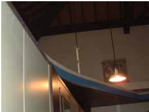
Old rail support that used to support the railing for the old suspended track.
