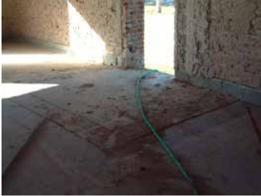
Original west entrance. The stairs that used to be here were filled in by concrete.
